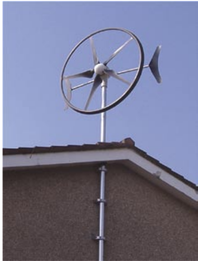
Figure 7 - School turbine installed at Collydean Primary
